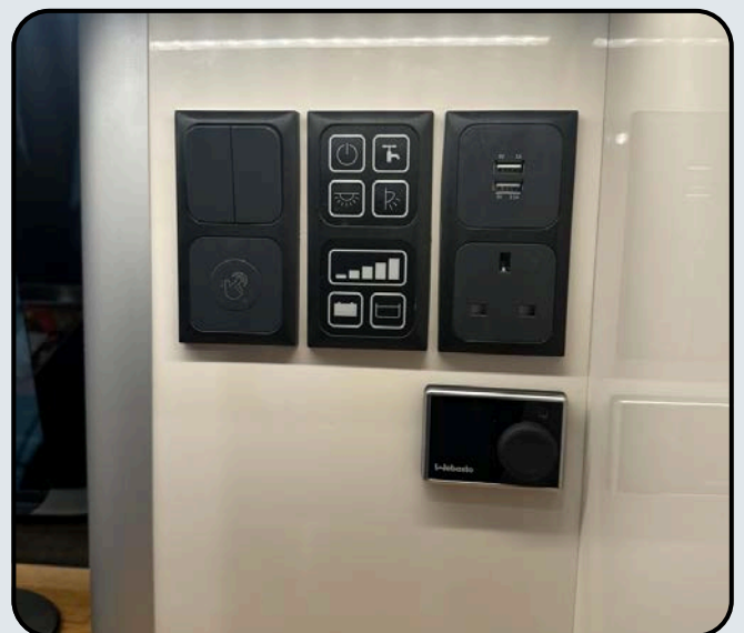
Vegas Button Control Panel
